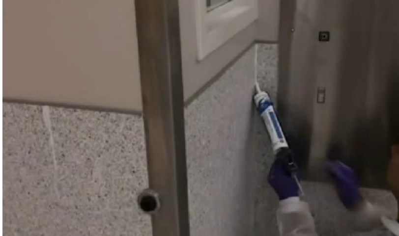
Photo #3: Use color-matched caulking to seal wall seams
